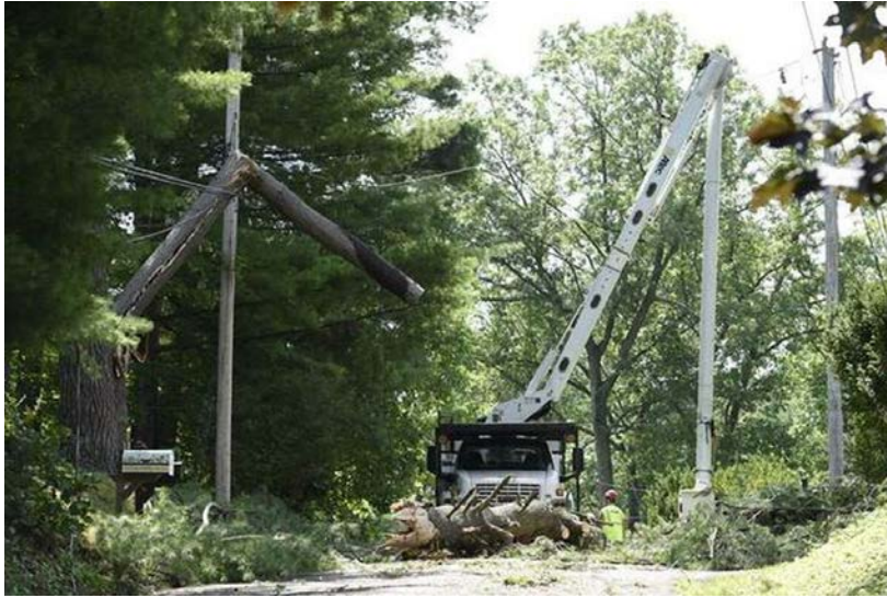
Figure 12. Damages caused by Extreme Storms in Columbia County (Image by Skip Dickstein/Times Union)
